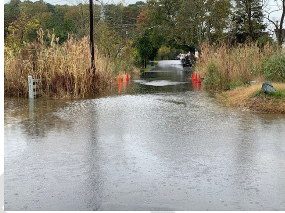
Photo 2 - Flooding at Grace Street Culvert
