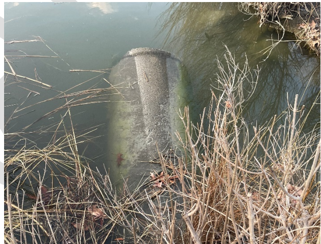
Photo 24 - Outfall Pipe from Retention Pond at W. Chestnut St. and Tilden St.
