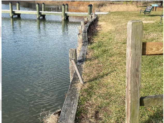
Photo 29 - Failed Bulkhead along Back Creek Park
