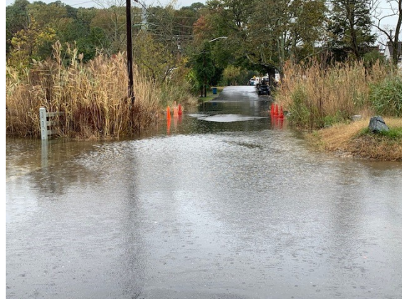
Photo 2 - Flooding at Grace Street Culvert
