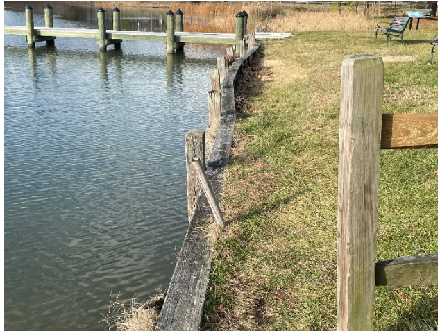
Photo 33 - Failed Bulkhead along Back Creek Park
