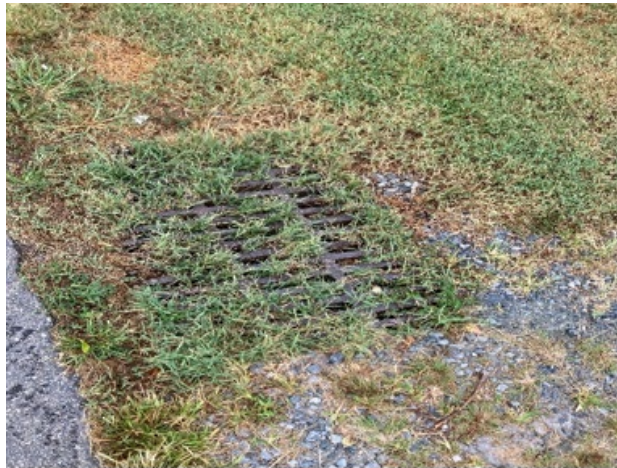
Photo 53 - Sedimented and overgrown inlet
