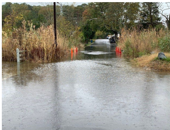
Photo 2 - Flooding at Grace Street Culvert
