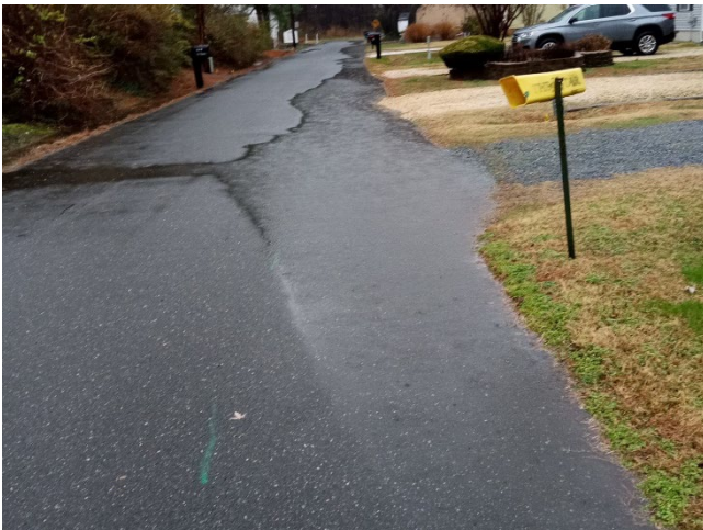
Photo 51 - Water ponding on road surface
