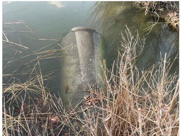
Photo 28 - Outfall Pipe from Retention Pond at W. Chestnut St. and Tilden St.
