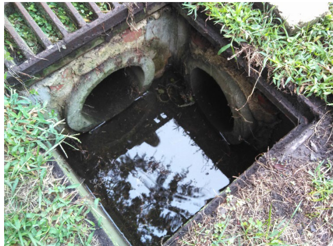
Photo 52 - Flooding of storm drains
