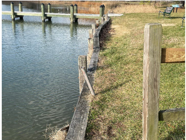
Photo 33 - Failed Bulkhead along Back Creek Park
